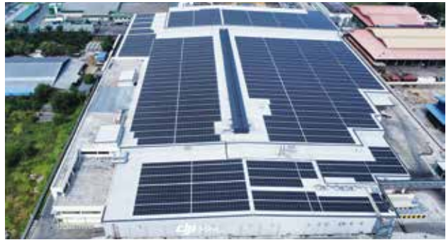
Solar Panel on the roof top of the Rendering Plant
