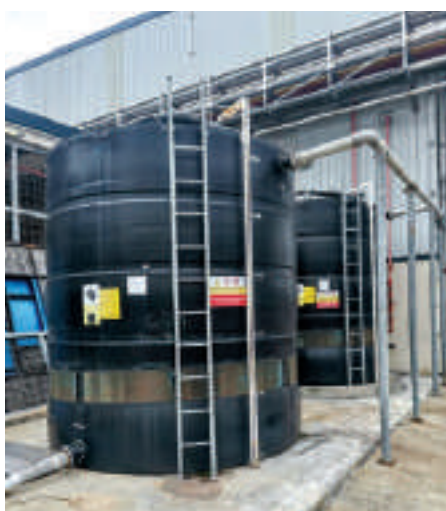
Harvested Rainwater Tank
